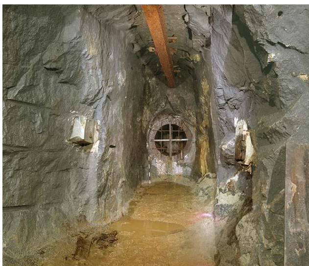
Ventilation fan and trunking installed during the AWRE period
